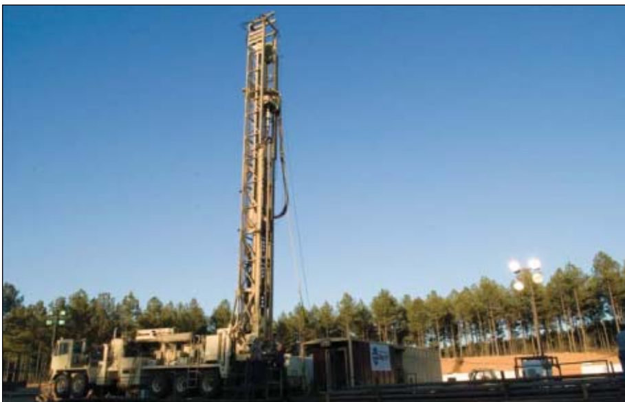
DeSoto Rig 31 drills top holes in the Fayetteville shale for Southwestern Energy (Fig. 3; photo from Atlas Copco Drilling Solutions LLC).
