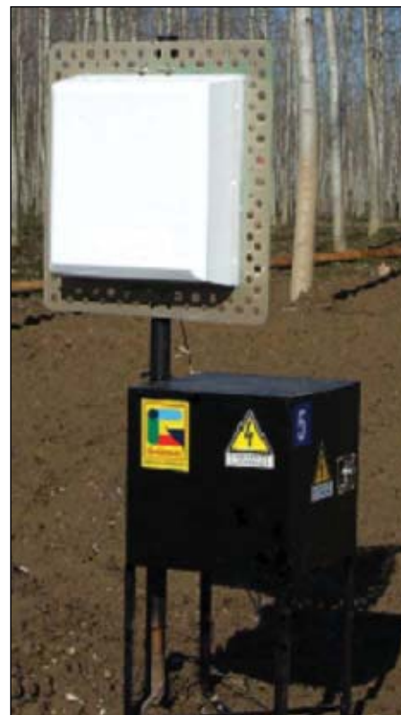
Radio thermocouple units are arrayed in the proper configuration to deliver data to a centralized control and gathering hub (Fig. 3).
