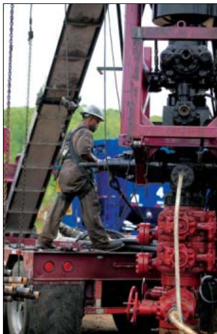
This crane was supporting a coiled tubing injector and wellhead in a Fayetteville shale drilling operation for Southwestern Energy in 2007 (Fig. 1; photo from Southwestern Energy).
